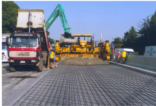
Fig. 25. A steel grid for the reinforcement of a new cement concrete highway in Belgium.
