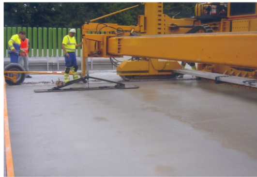
Fig. 22. The “super-smoother”, used for the smoothing of wet cement concrete making circular movements parallelly to the road axis, althuss avoiding undulations in the cement concrete surface.
