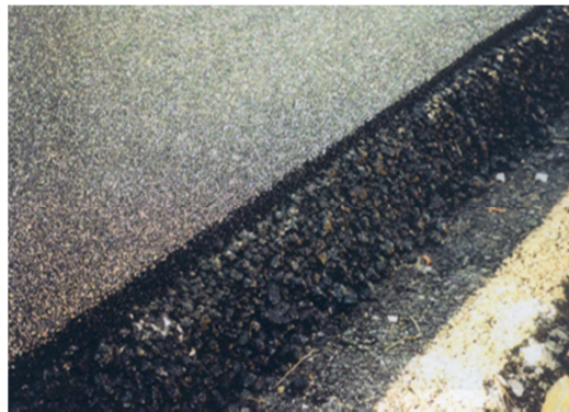
Fig. 18. Two layer porous asphalt with a 4/8 top layer (25 mm thick) and a 0/16 porous sub layer (45 mm thick).
