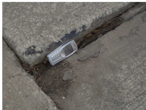
Fig. 16. Level difference between two non dowelled concrete slabs.
