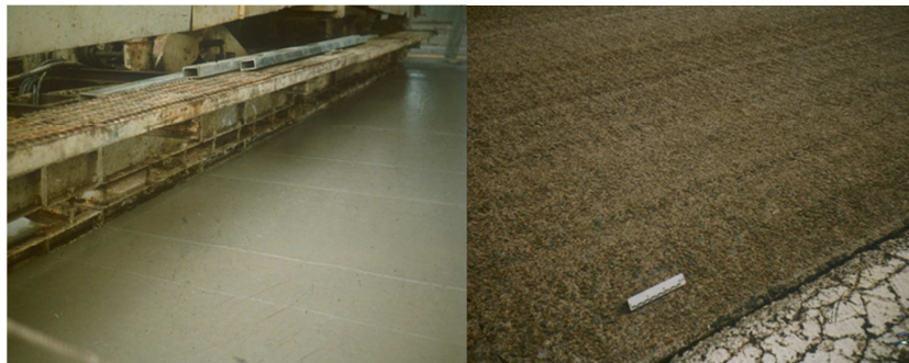
Fig. 15. Laying of a cement concrete surface with a classic screed, perpendicular to the road axis, leading to the quite common undulations, making the pavement extremely noisy.
