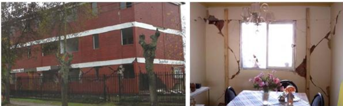
Figure 3: Damage in CM building due to the 2010 Chile earthquake (Brzev et al., 2010)
