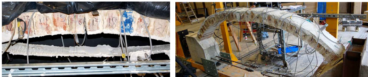
Fig. 11 Debonding of SRP applied at intrados (left) and arch reinforced at extrados (right) [16]
