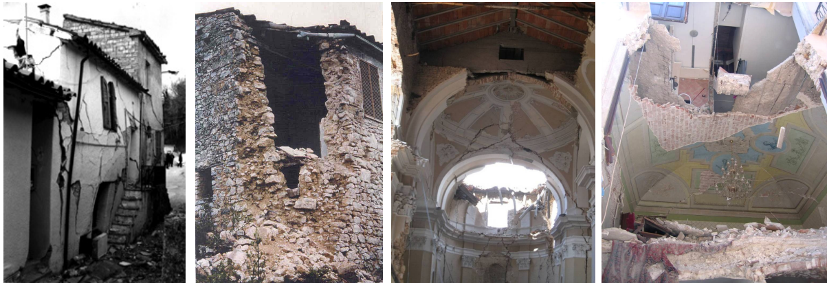
Fig. 1 Out-of-plane deformation due to lack of connection at intermediate floor level (left) and brittle collapse of corner (right), showing inadequate floor and roof (from 1997 Umbria-Marche earthquake, Italy) [6]
