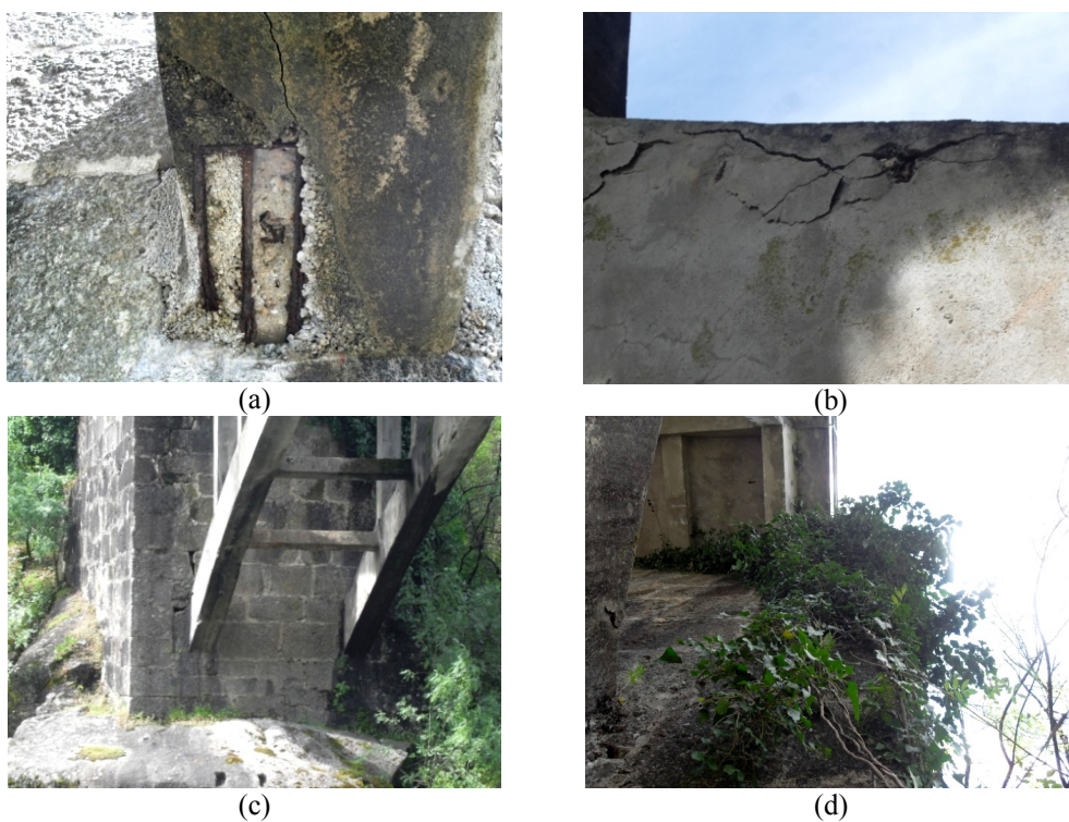
Fig. 6 (a) Corrosion of the steel reinforcement and loss of concrete cover due to spalling (b) Concrete spalling; (c) Cracks in the masonry abutment; (d) Biological growth on the bridge
