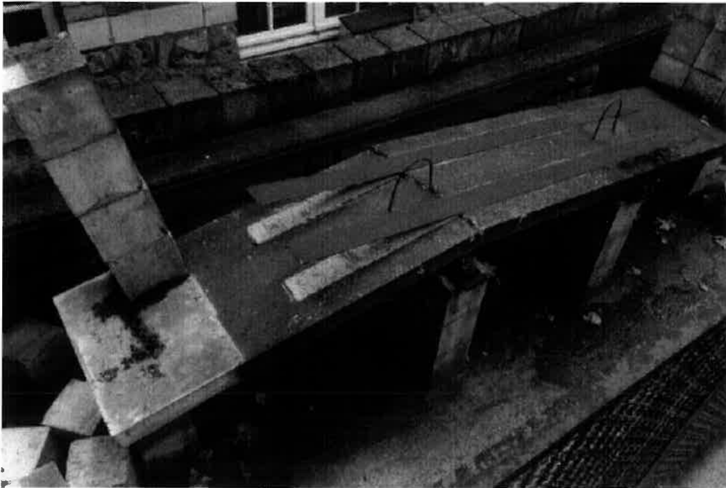
Figure 7: Strengthened plate, collapsed after 16 years of outdoor exposure
