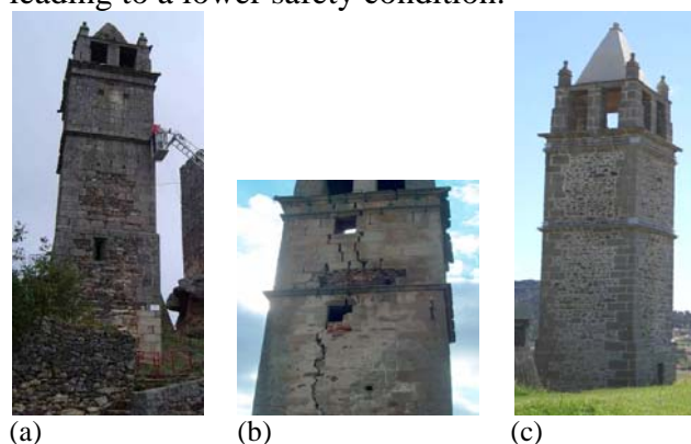
Figure 1 – Mogadouro Clock Tower: (a) and (b) general view of the tower with severe damage; and (c) the tower after the strengthening works
