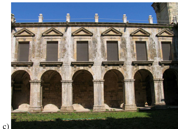
Figure 3. Actual monastery: a) aerial view from south-eastern side; b) ground plan; c) façade of the main cloister after the preliminary conservation works.
