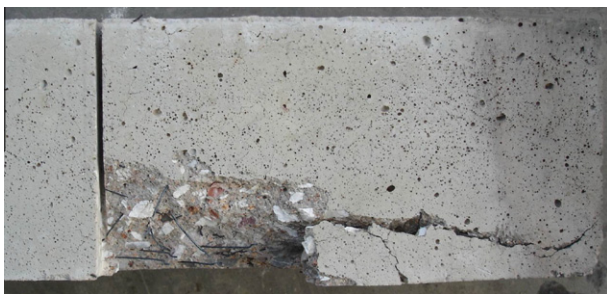
Fig. 11. Spalling of SF40 after 600 °C.
