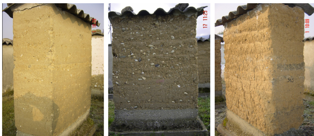
Fig. 3. Rammed earth masonry sections exposed during 20 years to natural climatic conditions. (a) Wall made with soil stabilized with 5% lime; (b) wall made with soil without stabilization (mixed soil); and (c) wall made with soil without stabilization [53].
