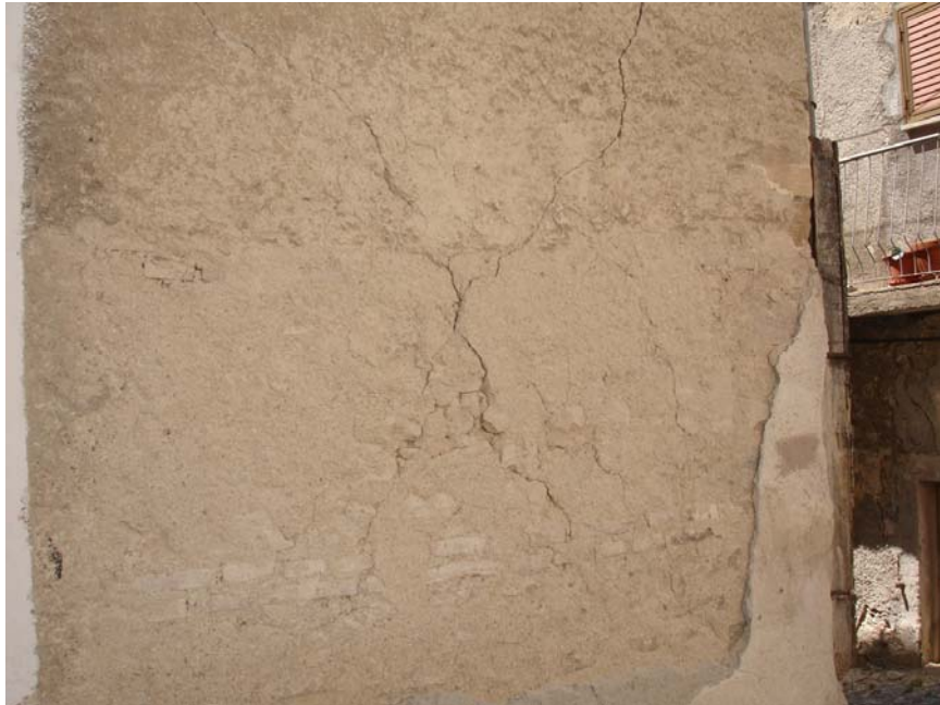
Fig. 2.13 Building located in the historical centre of Paganica. In plane behavior: the iron ties at floor level allowed the formation of diagonal struts in the masonry piers.
