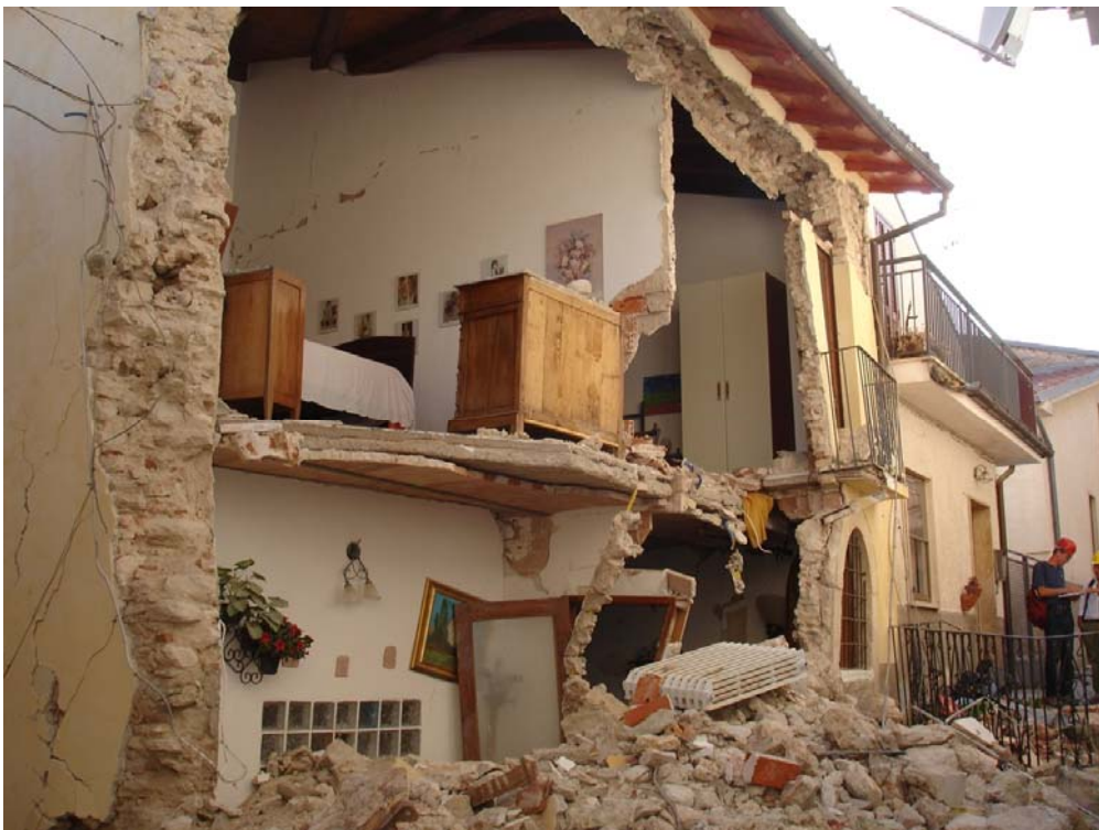
Fig. 2.9 Facade of a building located in the historical centre of Paganica. Out of plane behavior: flexural mechanism of facade wall. Note the inefficient connection of the wall to the roof, while the absence of iron ties made possible global overturning
