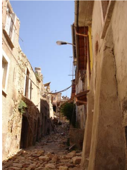
Fig. 2.10 Row of buildings located in the historical centre of Paganica. Out of plane behavior: collapse mechanism of the upper zone of the walls (left part). Note the poor quality of masonry, without efficient transversal connection elements, and the roof structure not well anchored to the wall. Iron ties avoided global overturning.
