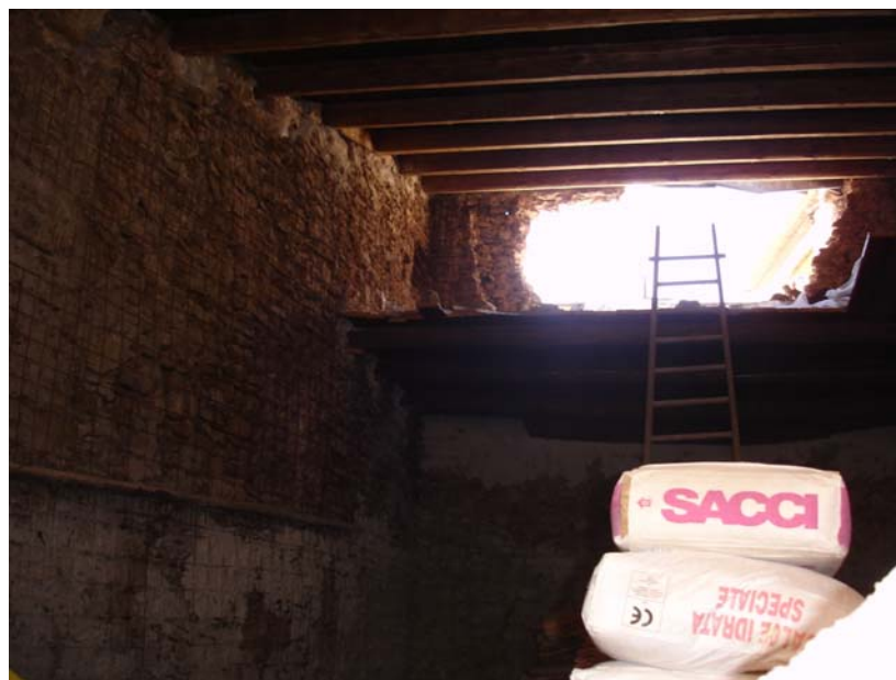
Fig. 2.11 Building located in the historical centre of Paganica. Out of plane behavior: collapse of the central zone of a wall determined by the horizontal action due to earthquake. The strengthened walls, a fair connection with the roof structure and iron ties avoided global overturning.
