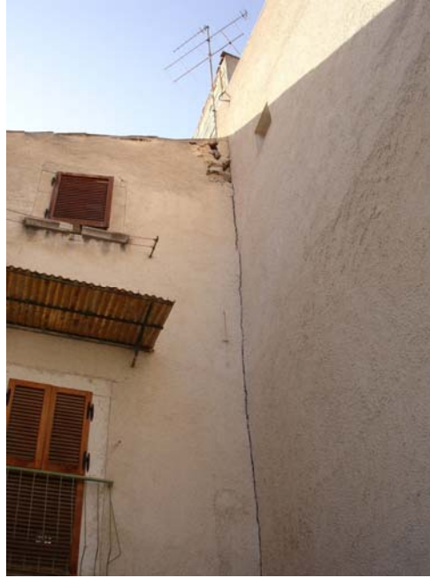
Fig. 2.16 Aggregates and complex buildings in the historical centre of Paganica. Damages due to different heights of adjacent buildings.
