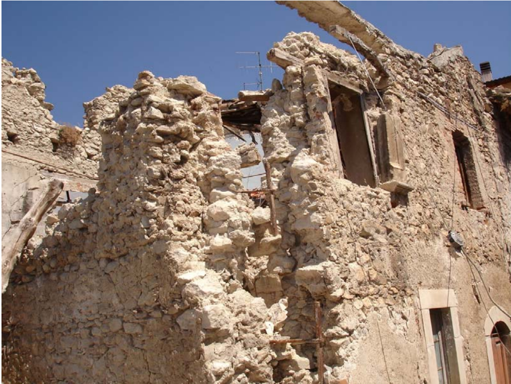
Fig. 2.14 Building located in the historical centre of Paganica. Global failure due to the poor quality of the masonry material. In plane and out of plane failure modes are visible. Presence of out of plane instability with expulsion of the corner between perpendicular walls.
