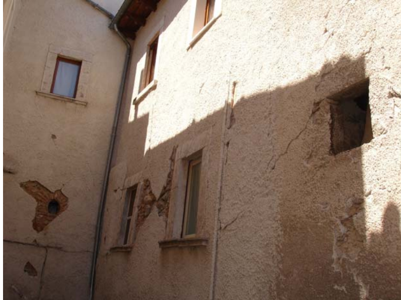
Fig. 2.12 Building located in the historical centre of Paganica. In plane behavior: several iron ties, placed in correspondence of orthogonal walls at each storey, avoided the out of the plane collapse. Diagonal cracks, in both spandrels and piers, demonstrate the engagement of the wall in its own plane.
