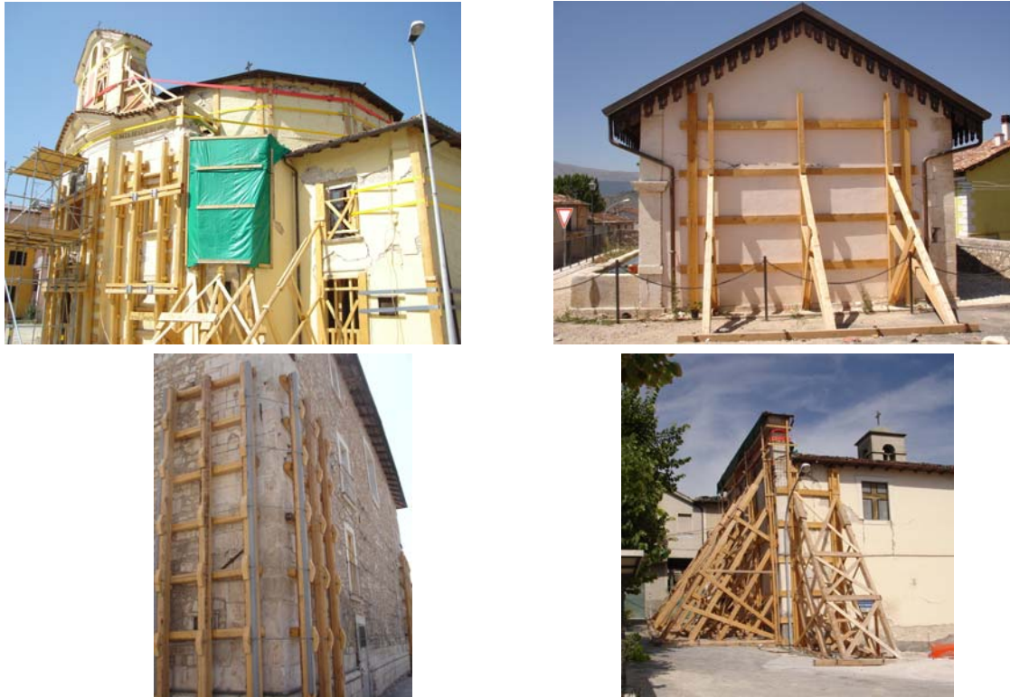
Fig. 2.6 Several wood frames and iron ties, placed after Aquila's earthquake, avoided out of the plane global failure of external walls, which resulted very damaged in their own plane. The cracks in the masonry walls demonstrate the strong engagement of these structural elements in the global response.
