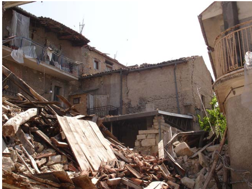
Fig. 2.7 Ancient masonry of a building located in the historical centre of Paganica. Out of plane behavior: separation between two orthogonal masonry walls due to poor arrangement of the stones.
