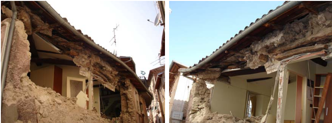
Fig. 2.8 Facade of a building located in the historical centre of Paganica. Out of plane behavior: flexural mechanism of facade wall. Note the inefficient connection of the wall to the roof, while iron ties avoided global overturning of the bottom part.
