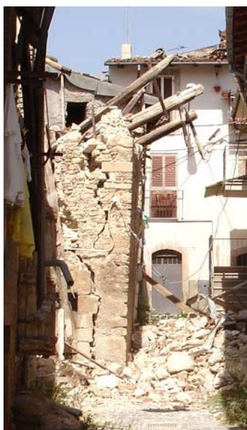
Fig. 2.5 Building located in the historical centre of Paganica. Out of plane behavior: overturning mechanism of the facade wall detached from orthogonal walls.
