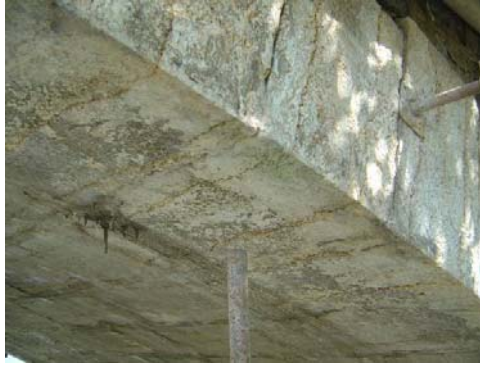
Fig. 3.42 Visual inspection: vertical cracks in the masonry blocks
