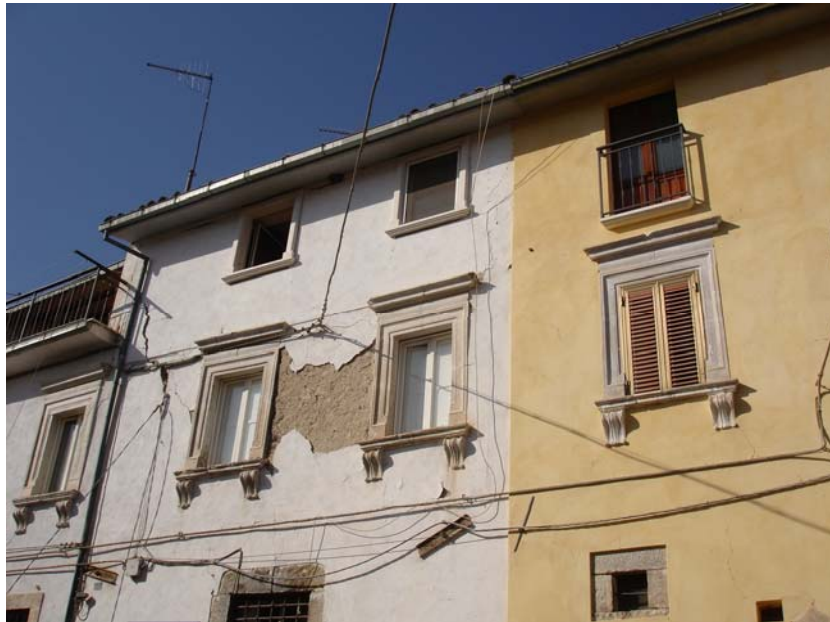
Fig. 2.15 Buildings located in the historical centre of Paganica. Good behavior of masonry buildings in presence of ancient iron ties: only some negligible diagonal cracks are visible on the spandrels.
