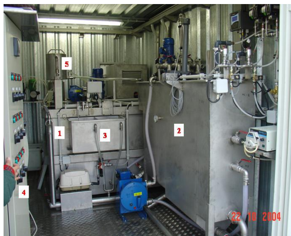
Figure 1. Image of the pilot Hybrid Membrane Bioreactor plant: 1.- equalization tank; 2. Membrane Bioreactor; 3.- Permeate tanks, 4.- Control panel; and 5 Fine screen
